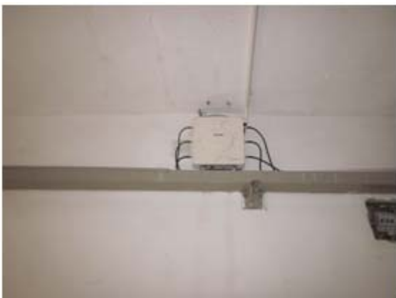
Figure 3-5 Real-World Application of i-Share Solution
